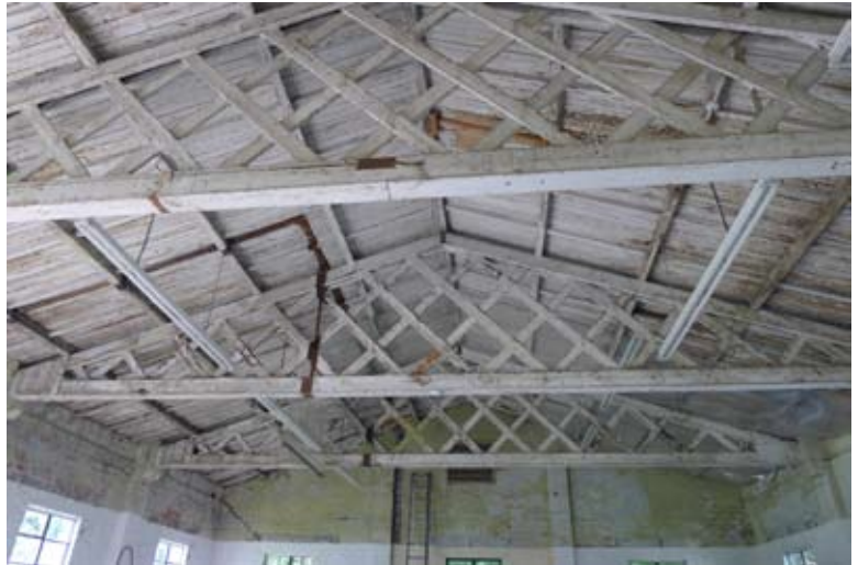
Fig 6. Wooden lattice Belfast trusses in the welders' shop (© English Heritage, photograph: Clare Howard)
