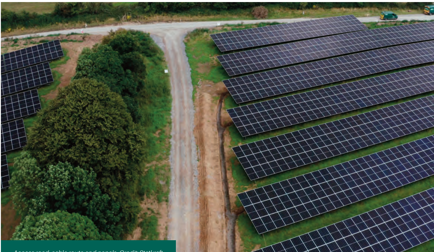
Access road, cable route and panels. Credit: Statkraft
