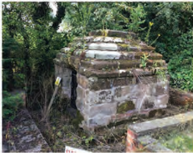
Stone 2 Asset Location: Stone Moor Farm Shropshire, 18th Century Proposed for excavation and reconstruction Owner: HS2 © HS2 Ltd
