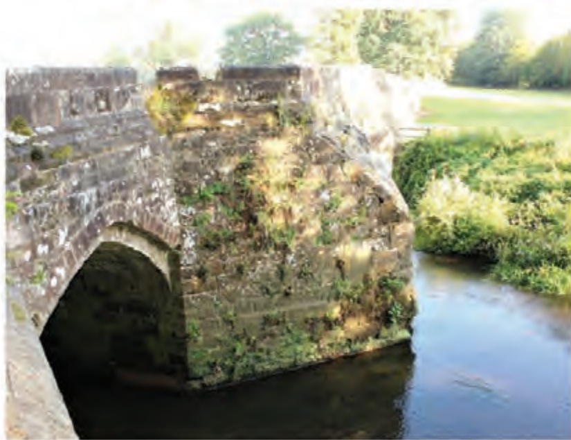
Scheduled and Listed 15th Century Stone Bridge, Stoneleigh Abbey Work is currently underway for crossing (Credit: HS2 Ltd)
