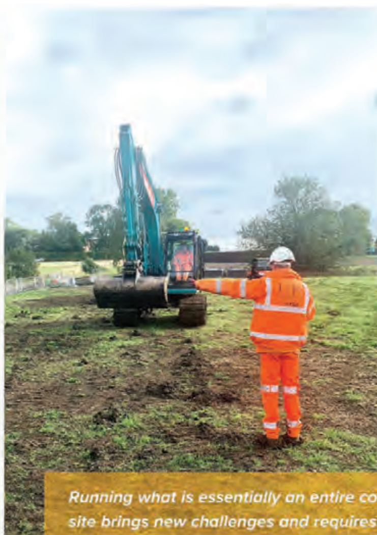
L – P: Archaeology staff working as bankspersons to safely oversee the movement of plant and delivery lorries. Credit: L – P Archaeology; © HS2 Ltd
