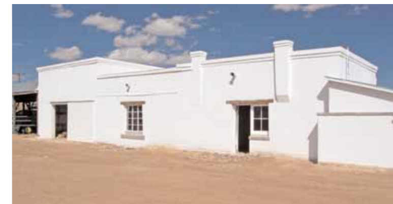
Canoa ranch buildings after conservation by Pima County © Simon Herbert, Pima County
