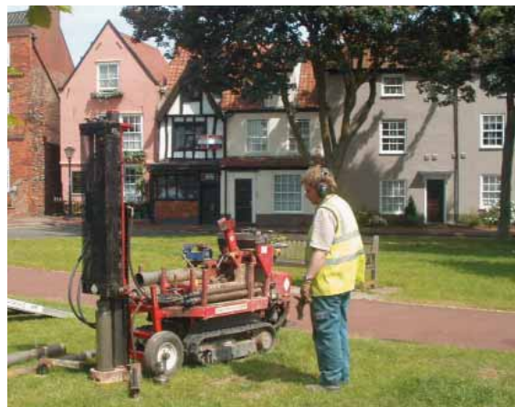
Borehole drilling for the Great Yarmouth deposit model outside Anna Sewell's house, Great Yarmouth. Photograph: Ken Hamilton
