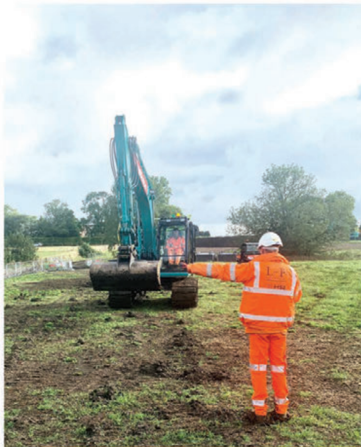
L – P : Archaeology staff working as bankspersons to safely oversee the movement of plant and delivery lorries. Credit: L – P Archaeology; © HS2 Ltd
