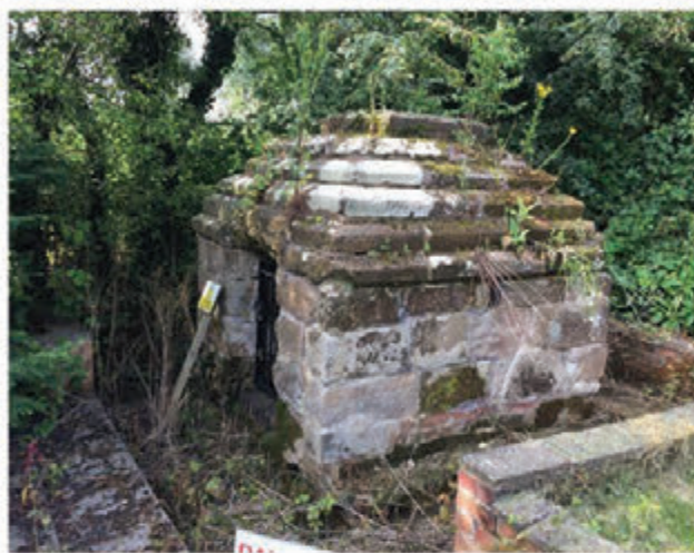
Grade 2 listed plunge bath at Manor Farm, Streechay, 18th century (monitored for cracking and water level drop). Credit: WSP; © HS2 Ltd
