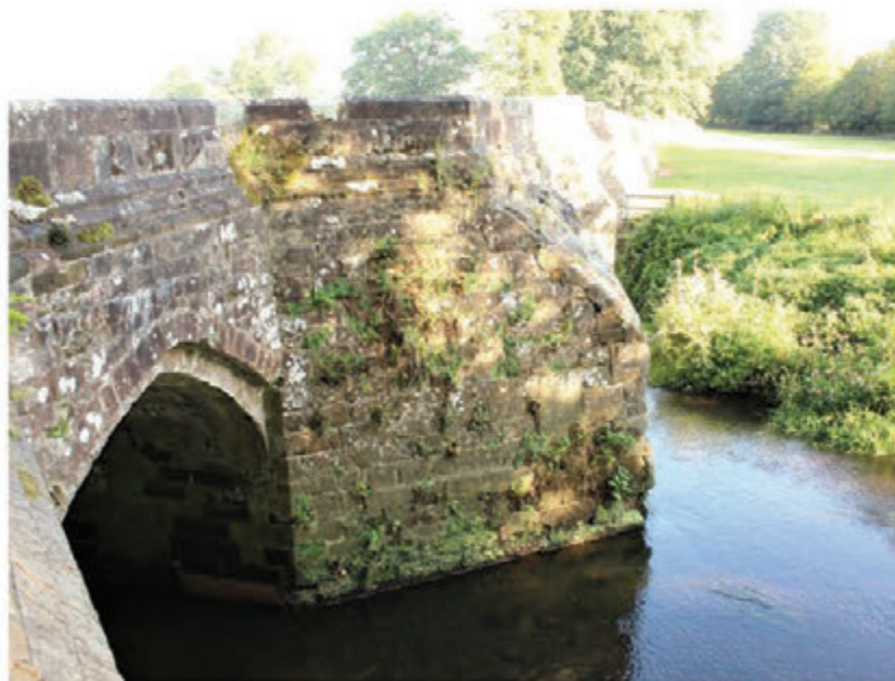
Scheduled and Grade 2* listed Stare Bridge, Stoneleigh Abbey, 15th century (monitored for cracking) Credit: WSP; © HS2 Ltd
